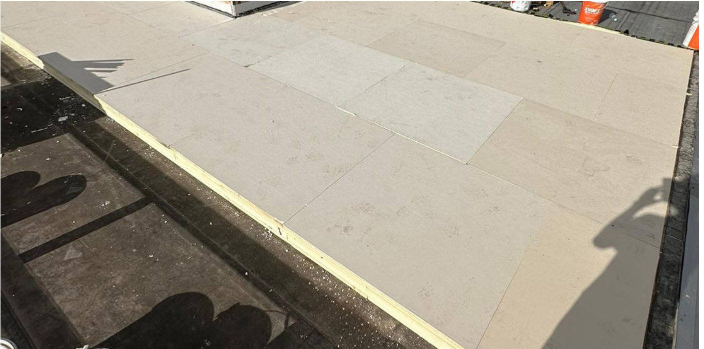
GREEN ROOF INSULATION
